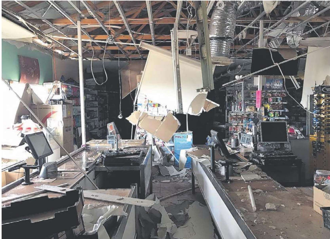
A storm caused extensive damage to the inside of the store. Picture: Wiluna Traders
